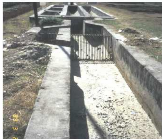
Photo 2: A Few Years Later: Out of Operation (due to the fact that the complementary institutional framework was not established and no funds were available for maintenance
